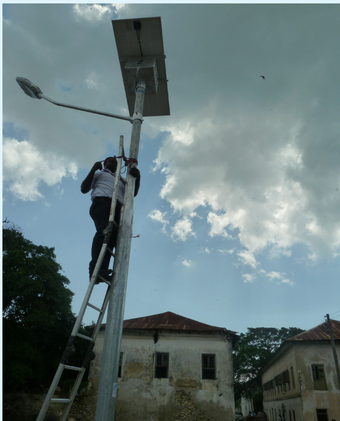
Installing the solar lights in Bagamoyo, an activity under the EMS/TEST thematic area (Photo: COAST Project)
