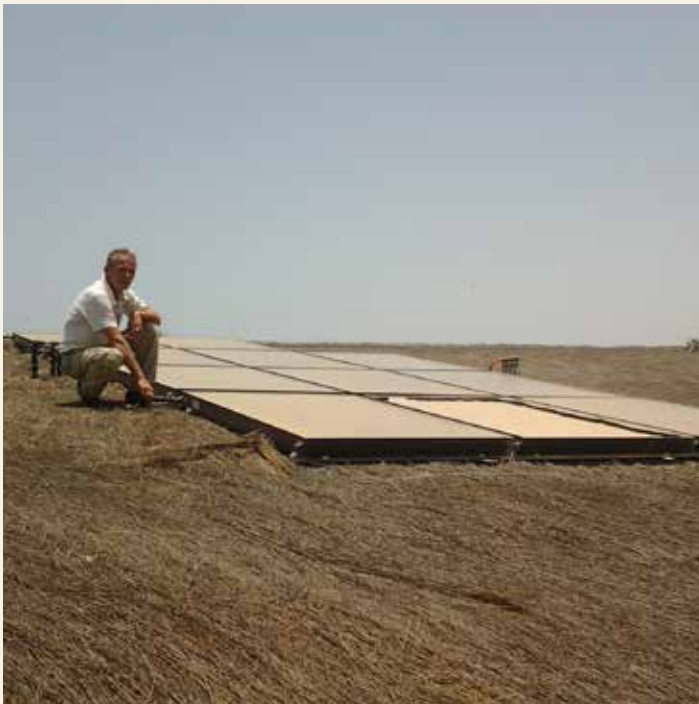
Mr. Martin Schmitz, Technical staff of the Lamantin Hotel, with the solar panels located on the roof of the hotel that are used to heat water for the hotel (Photo: COAST Project)
