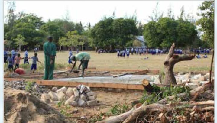
The construction of the platform for the water plant is now complete. The water equipment installation is expected to commence at the earliest opportunity (Photo: COAST Project)
