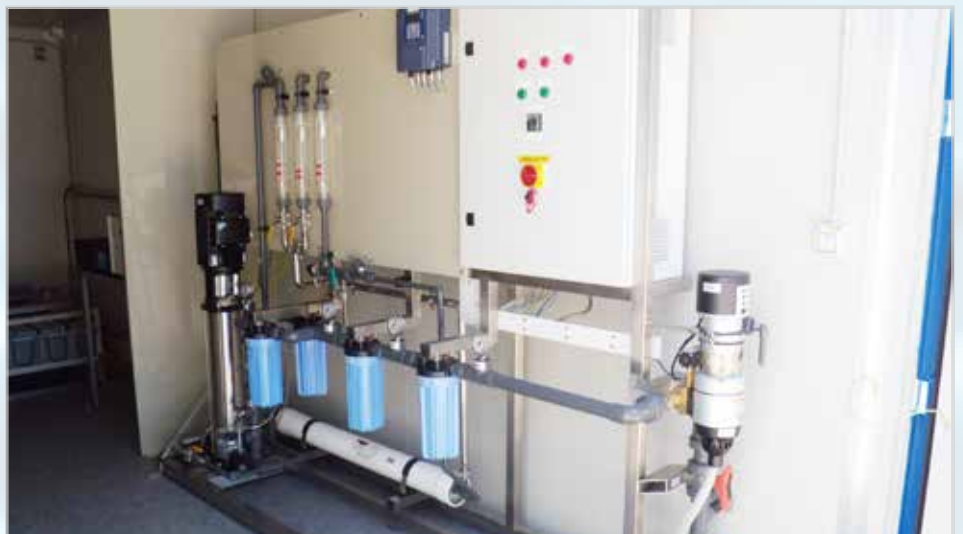
A picture of the water treatment equipment. The equipment utilizes reverse osmosis technology (Photo: COAST Project)
