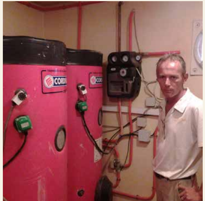
Mr. Martin Schmitz, showcasing the hotel solar water boilers that are used to heat the water in the kitchen and for the laundry services (Photo: COAST Project)
