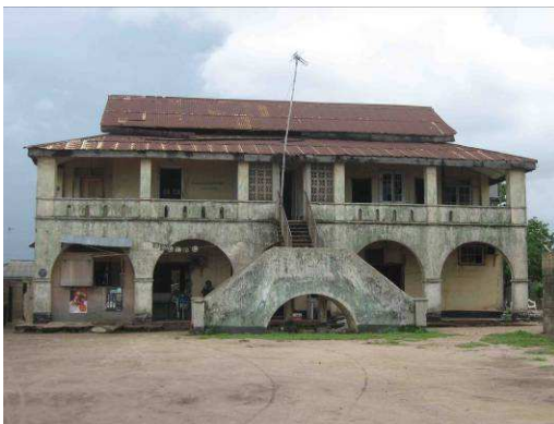
Photo 7: Decaying former District Officer's residence
